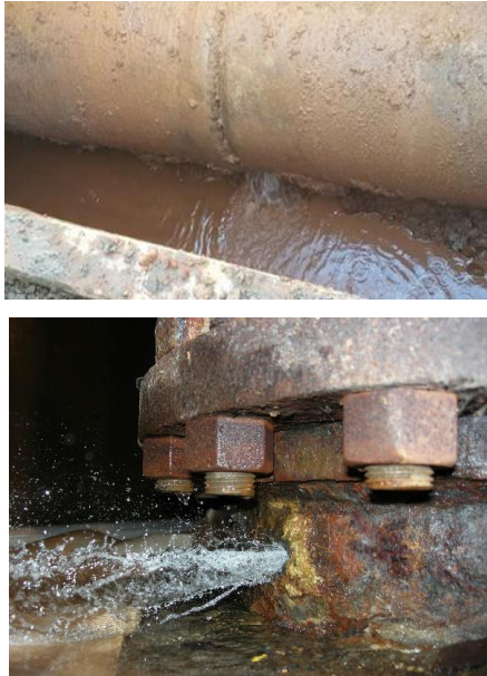
Figure 1 Examples of pipework failures
